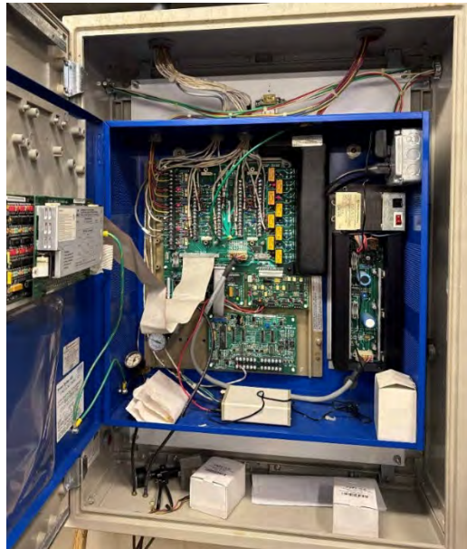
Local Control Panel
