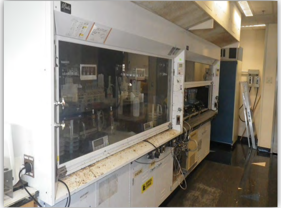
Typical Fume Hood
