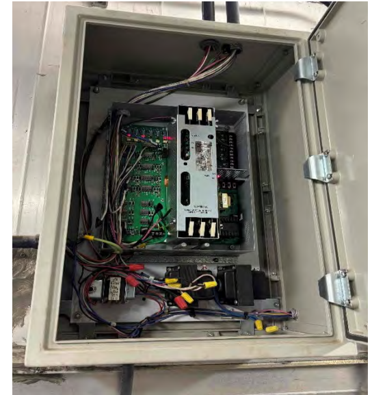
Local Control Panel
