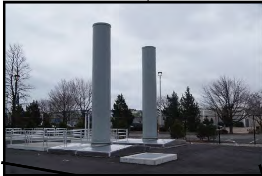
North Dorchester Bay Odor Control/Ventilation Facility
