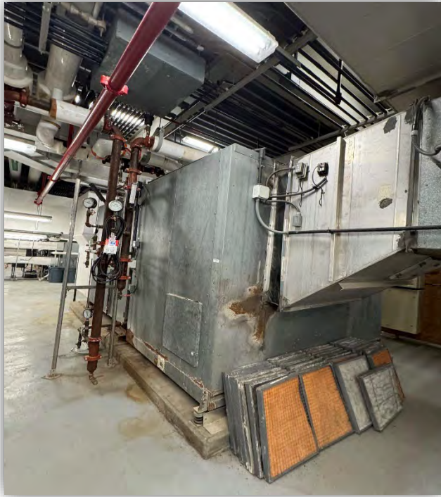
Typical HVAC Unit
