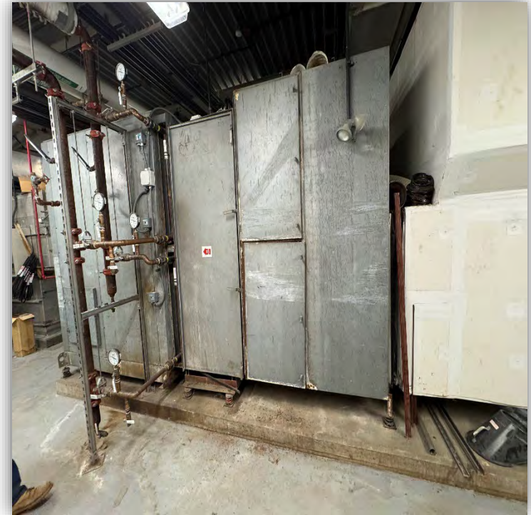
Typical HVAC Unit
