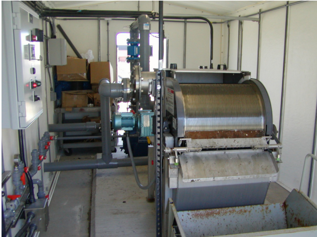
Figure 6-1. Effluent floatables sampling device. Samples were collected at the end of the west disinfection basin, after the final tip tube and scum baffle, prior to discharge to the outfall.
